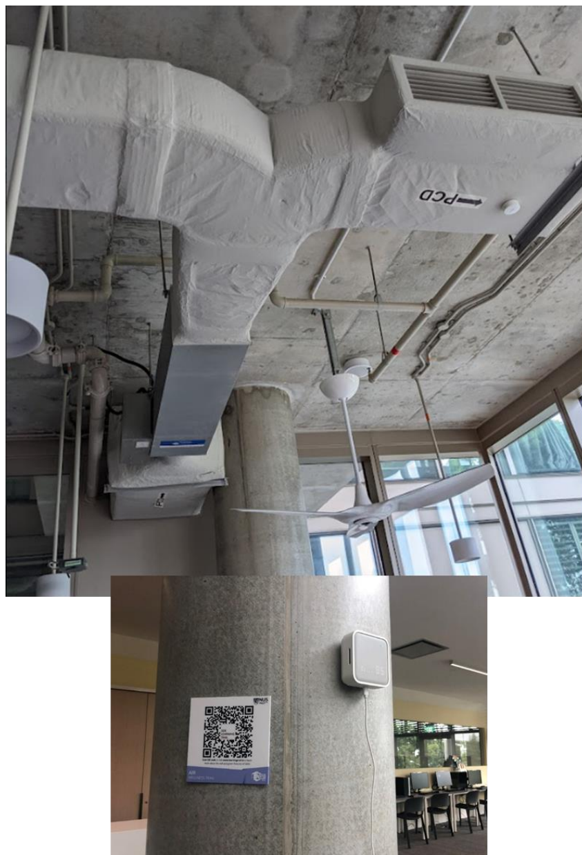
Figure 89 - NUS SDE4 Mechanical Ventilation and Ceiling Fan, & IAQ Sensor photos
