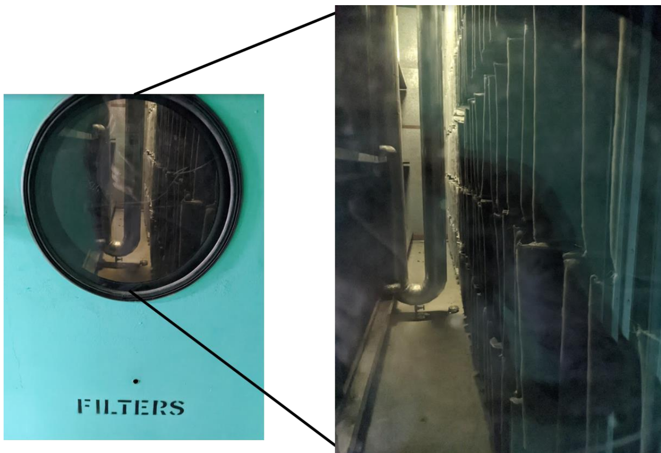
Figure 100 - 161 Collins Street AHU Filters
