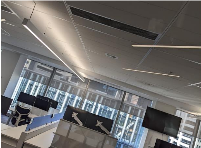
Figure 104 - 20 Martin Place Office Ceiling Supply & Extract grilles
